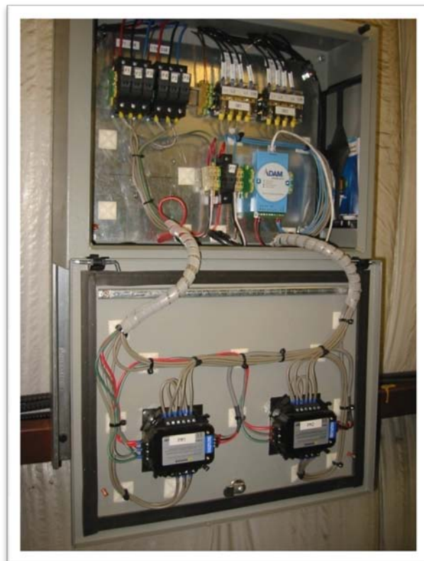
Electrical metering at Flakeboard’s St. Stephen plant. Photo courtesy of Flakeboard.
