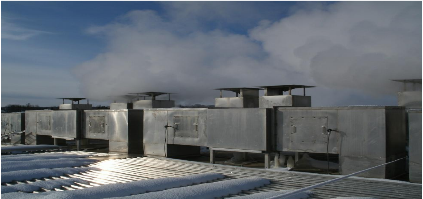
Heat recovery from exhaust on roof of new kilns
